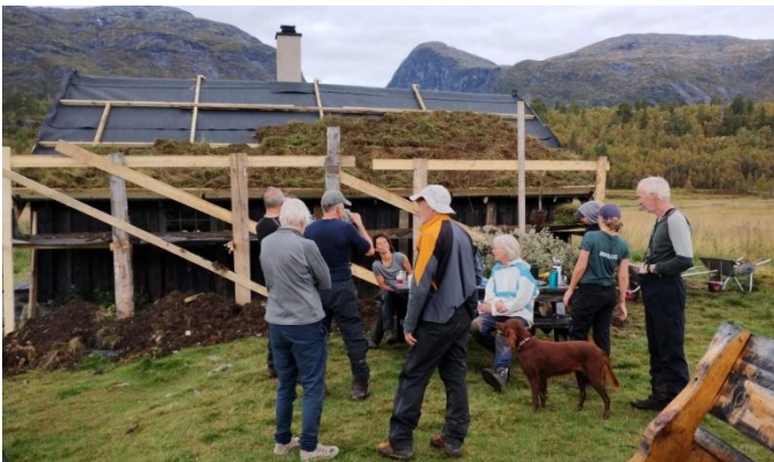
A tea break for the roof turfing party, Helen left, Kjetil right
